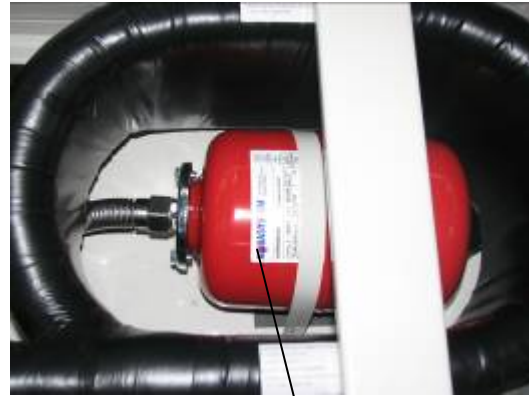
Expansion gas tank
